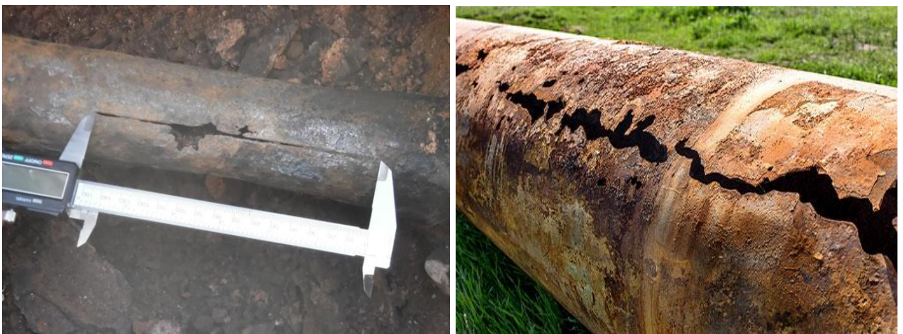
Figure 39 : Corrosive attacks on the external wall of a metal pipe
