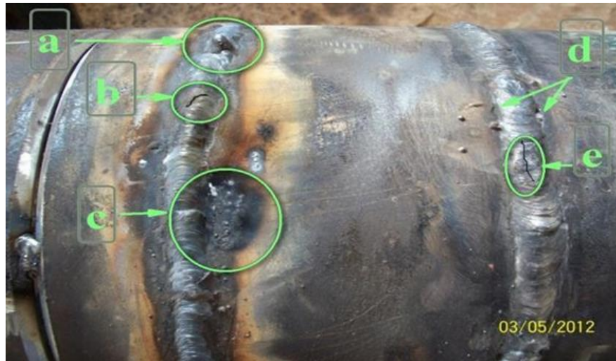
Figure 42: Weld seam with defects (crater, bites/channels, crack, Arcing initiations). [11]
