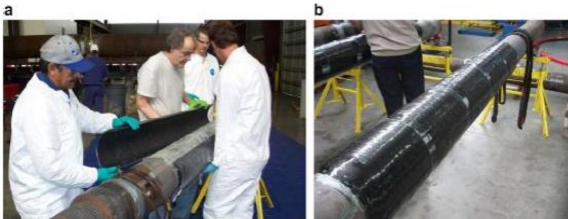
Figure 52 : composite patches repair
