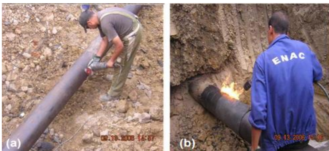
Figure 51: (a) surface repair for recoating, leakage of benthalha (Oran, Algeria), (b) re-coatin
