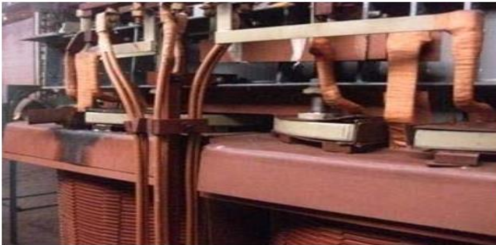
Figure B.3: Illustration of a real case of loose clamping structure
