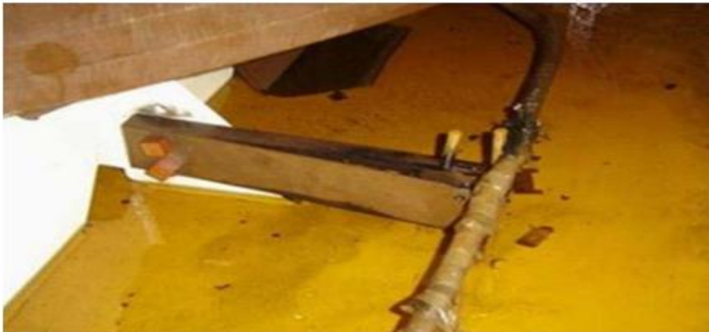
Figure B.8: Illustration of a real case of failure to ground
