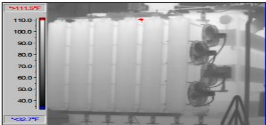
Figure 3. 12: IR for Transformer Tanks
