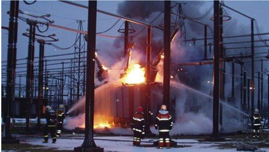
Figure 1.8: An oil-impregnated paper (OIP) bushing failure on the 400-kV, 100-MVAR reactor caused this reactor fire an oil-impregnated paper (OIP) bushing failure on the 400-kV, 100-MVAR reactor caused this reactor fire [14].
