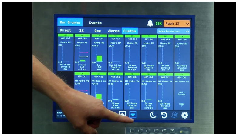
FIGURE 1.18: Bently Nevada 3500/94M Display HMI
