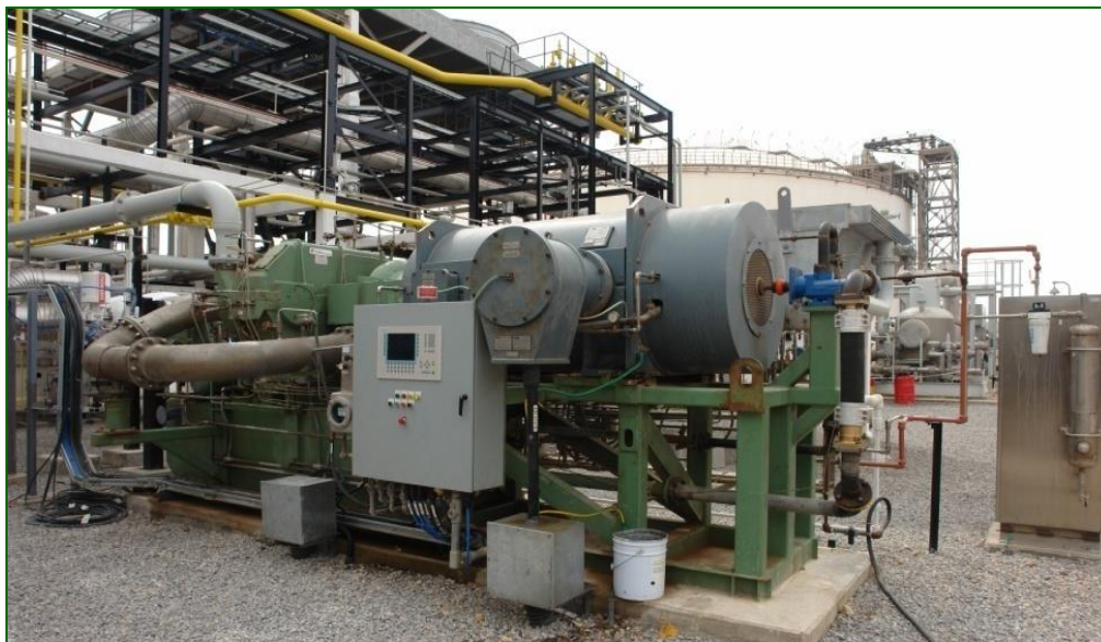
Figure III.6 : Compresseur Cooper BOG propane.
