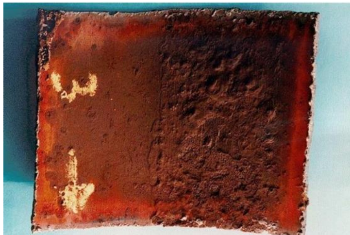
Figure II. 6: Pipeline corrodé intérieurement.
