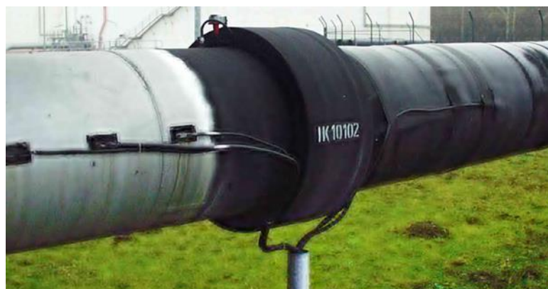
Figure II. 9: Un pipeline revêtu.
