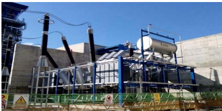
Figure [I.21] : Transformateur principale
