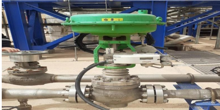
Figure [II.14] : Vanne de surchauffe
