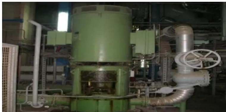
Figure [I.17] : pompe extraction
