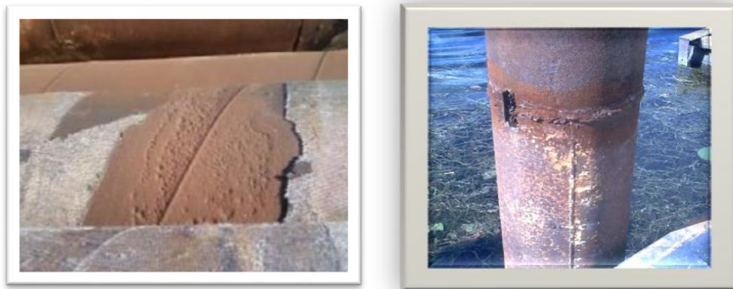
Figure I.1. La corrosion uniforme [10].
