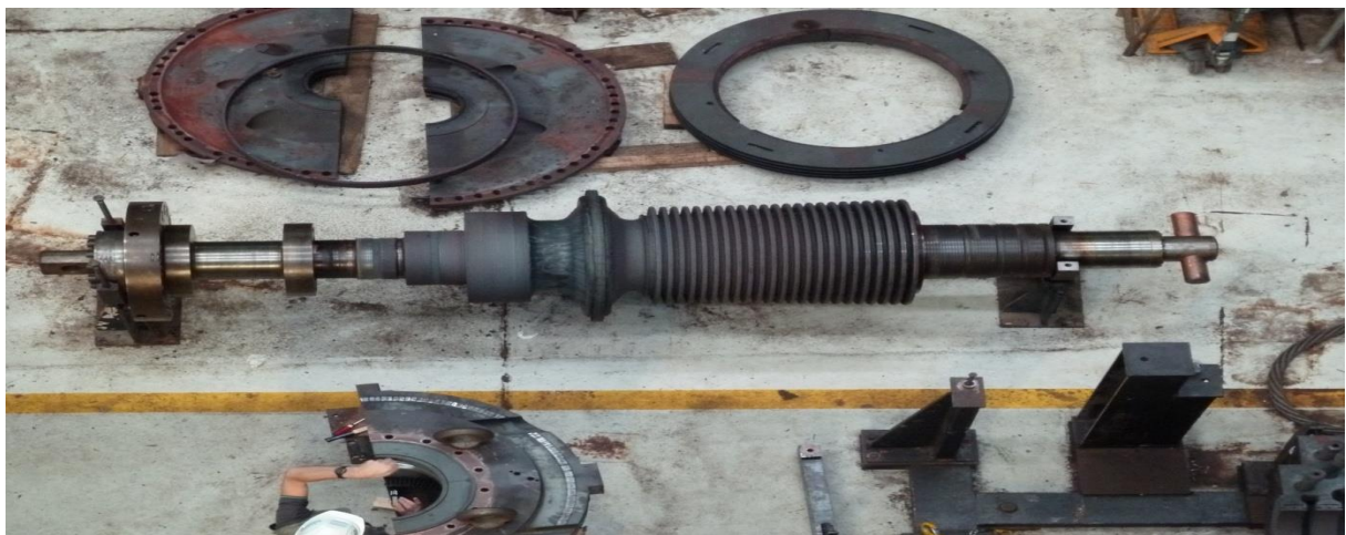
Figure I.6. Corps turbine haute pression (HP).
