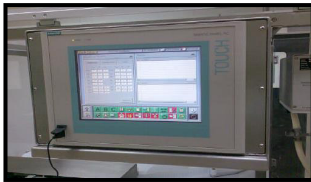
Figure II.2 : PLC (programmable logic Controller)
