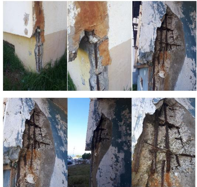
Figure 4. Degradations observed on the building.
