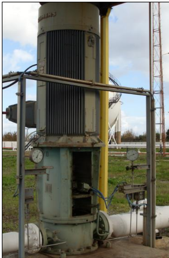
Figure II.7 : Pompe de transfert Blida.
