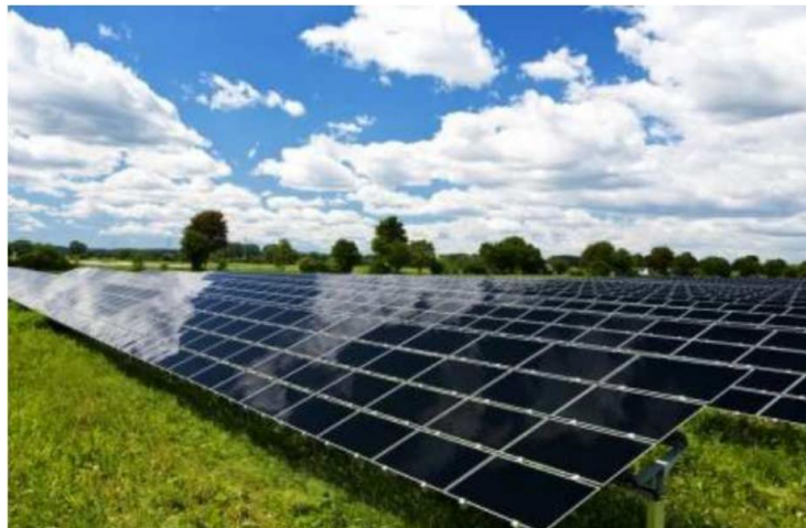
Figure 3.2: PV system under partial shading.
