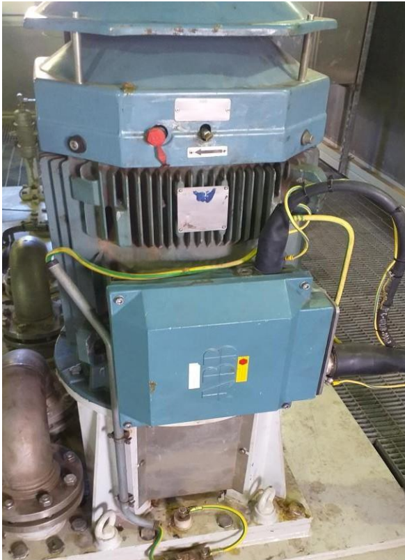
Figure II-12: pompe principale de lubrification
