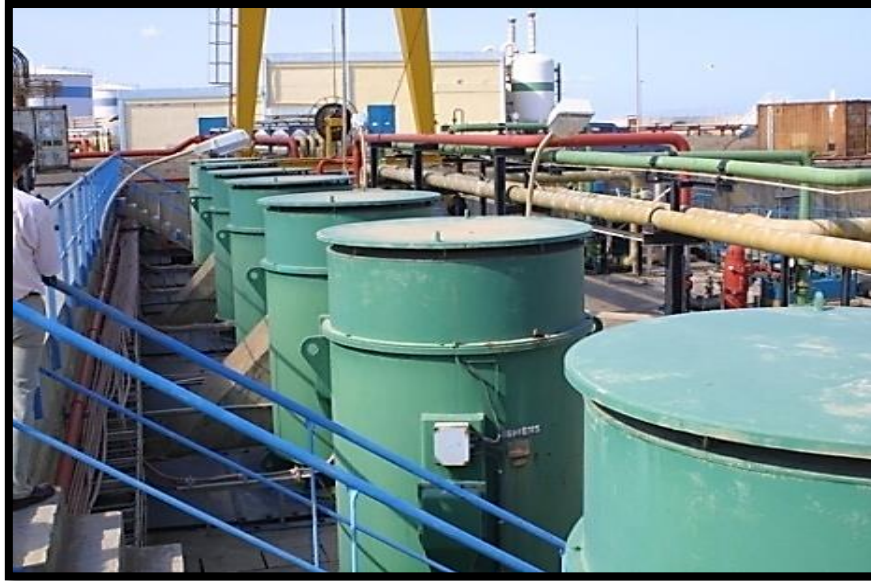
Figure I.8 : station de pompage.
