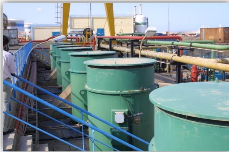
Figure I-9 : Station de pompage
