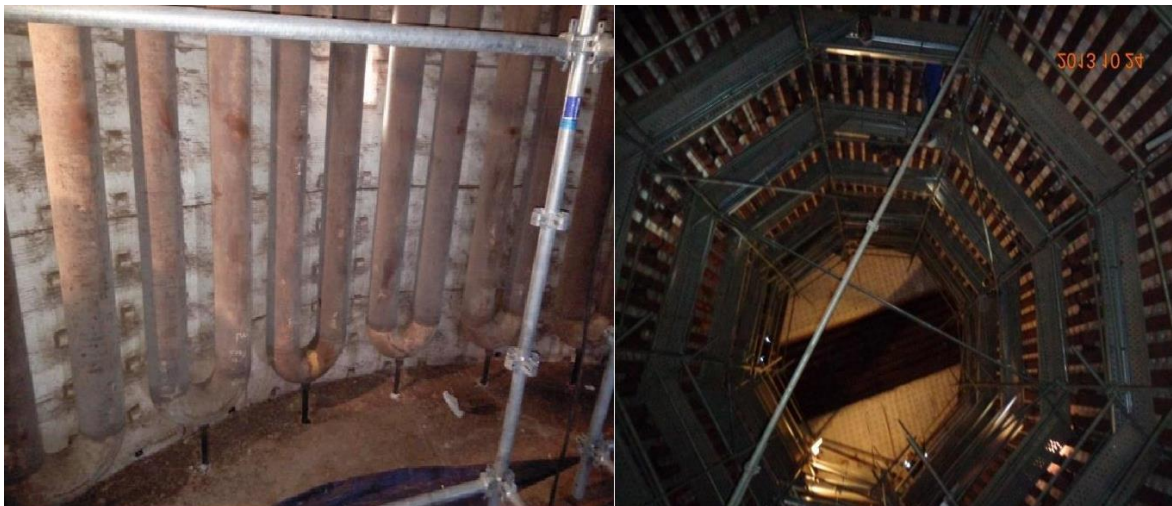
Figure 3-10 : Tubes verticaux de la zone de radiation Four RA2/K
