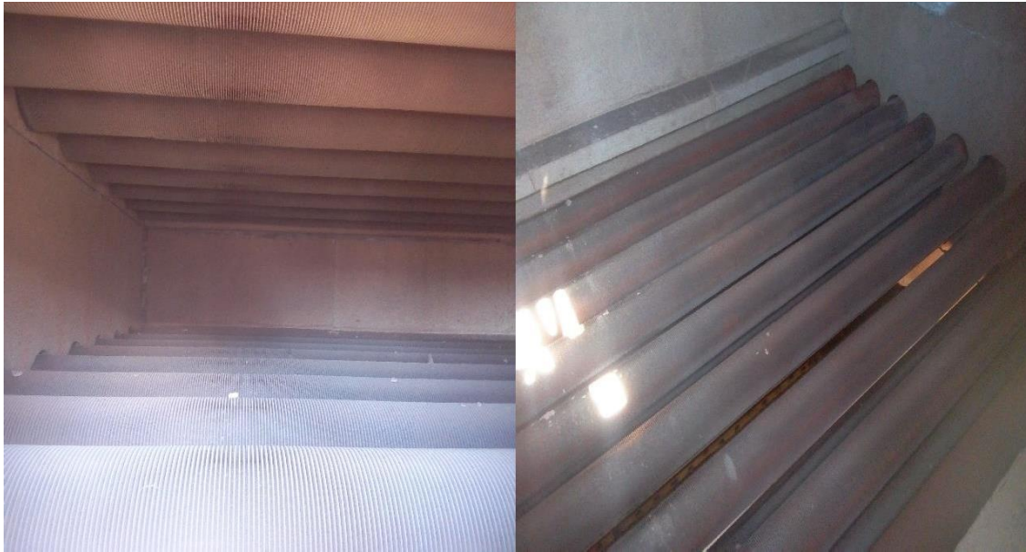
Figure 3-13 : Tubes ailettes de la zone de convection RA2/K
