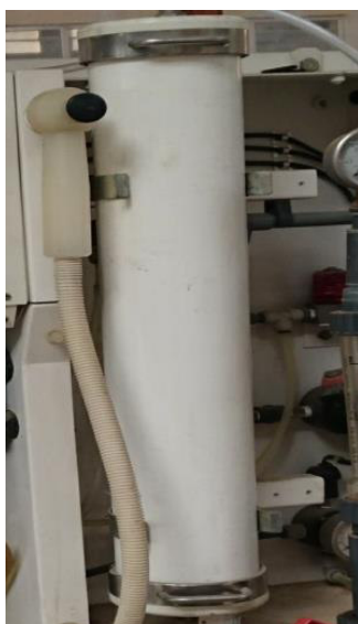
Figure 65. Membrane osmose inverse
