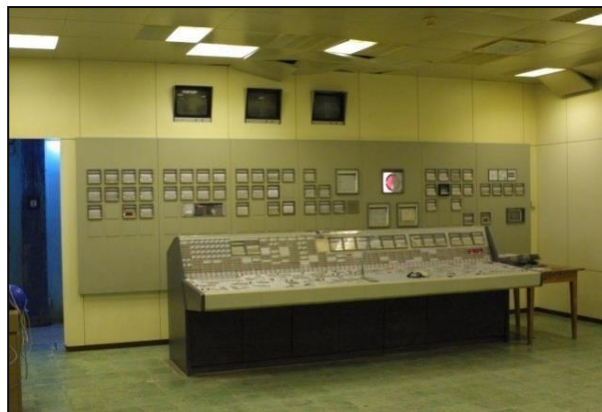
Figure (1.9) : Salle de commande. [2]
