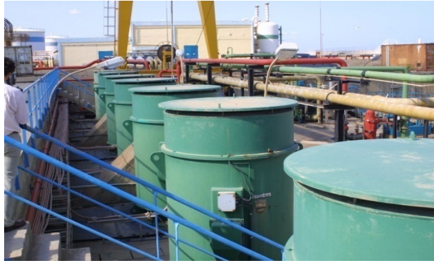
Figure I.11 : Station de pompage
