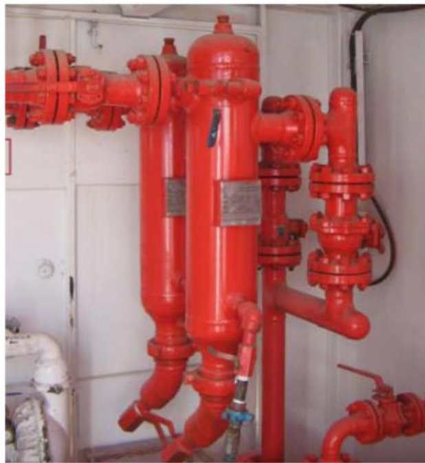
Figure 25 : Weatherford's Sample Catcher Unit.
