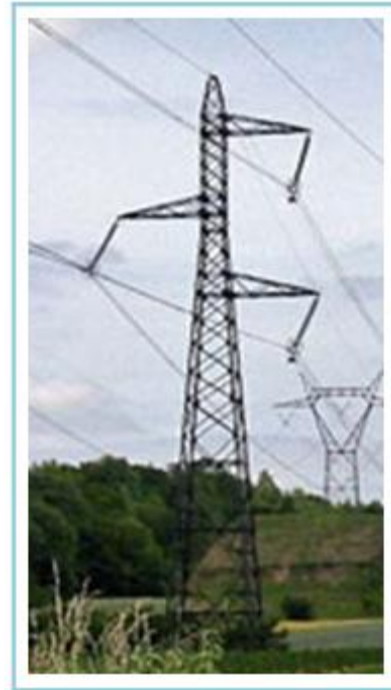
Figure (II-8): Pylône de type quinconce.
